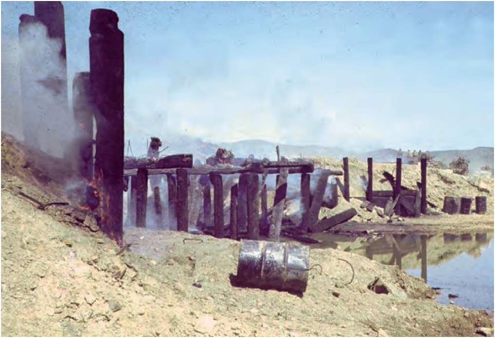
Before and during the Tet offensive, the Viet Cong consistently attacked bridges like this one burnt along Highway 1 north of Qui Nhon.
